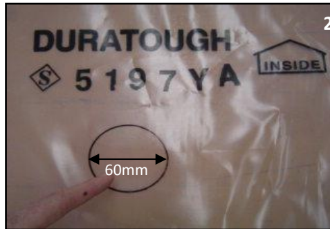
Mark a 60mm hole onto the inside twinskin cover at least 1 meter away from any of the films edges
