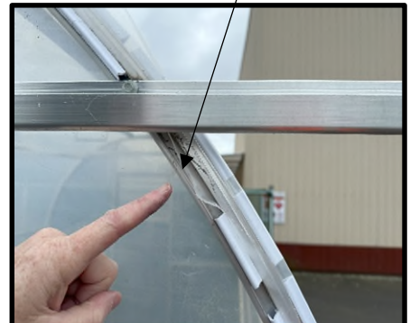
PicD3 Leave a piece of V-Lock out where the door slides past the end arch
